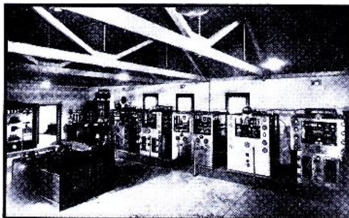
Transmitter room at A. W. A. Radio Centre, Braybrook, Victoria, where the transmitter of the short-wave station VK3ME is situated. This is the smaller of the two stations.
